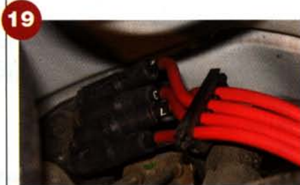
We installed the Power Cables one bank at a time, reattaching the stock separators along the way.
