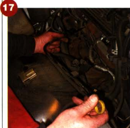
We also removed the dipstick by wiggling it out of the block.
